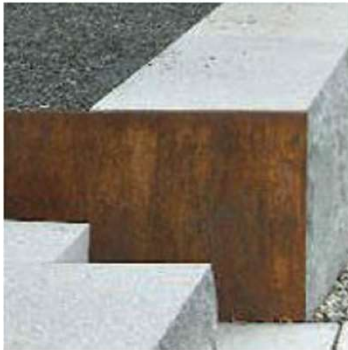
7. Steel Retaining Wall
